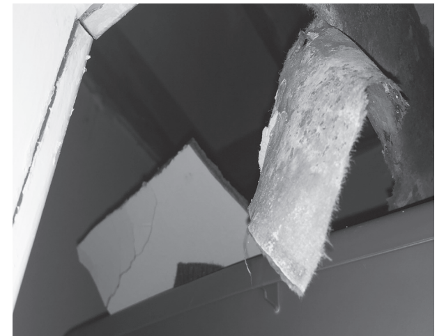
Water damage in a Venable closet that led to mold occurring (Photo: Logan Stum)
